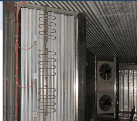
Heater electrical and hot water.
