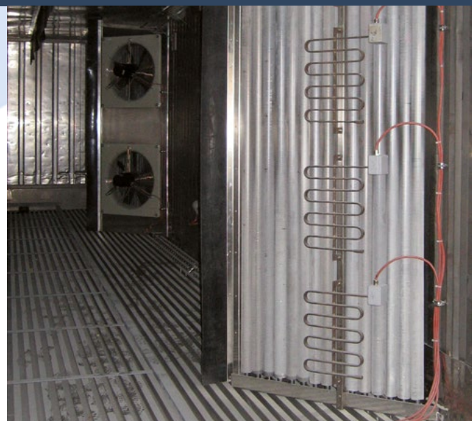
Heater electrical and hot water.
