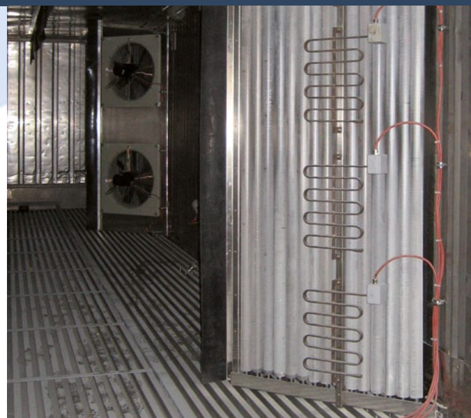
Heater electrical and hot water.
